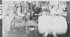
In top picture, Juan Tromp makes final connection for oil line to oil
